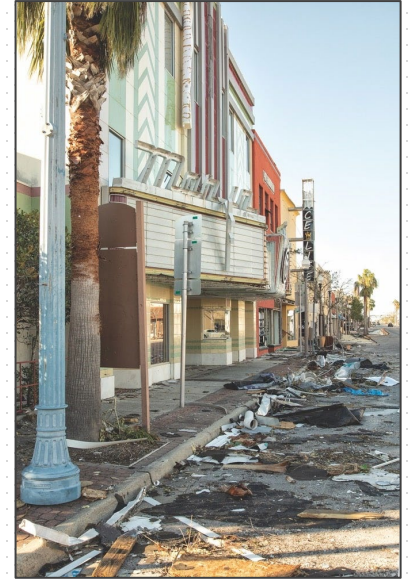
The Theatre was damaged during Hurricane Michael and has been closed to the public since. Photo credit: Jack Gardner
