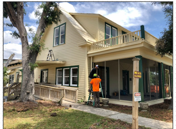
The McKenzie House is undergoing restorations and repairs in 2020. Photo credit: City of Panama City.
